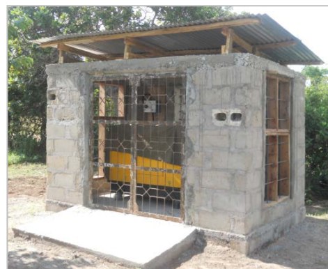
Generator and housing at Shirati EMBLEM
